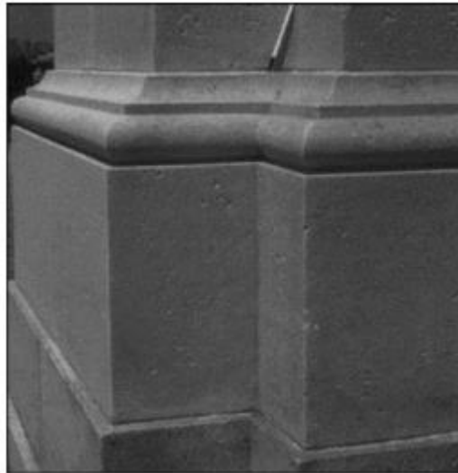
Figure 13 – Pock marks in marble column
