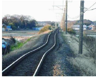
Picture 6 - Track settles differentially due to weak subgrade
