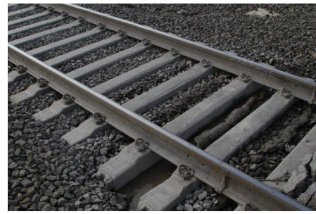
Picture 5 - Track fouls due to mud pumping
