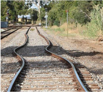
Picture 7 - Track buckles due to lack confining pressures
