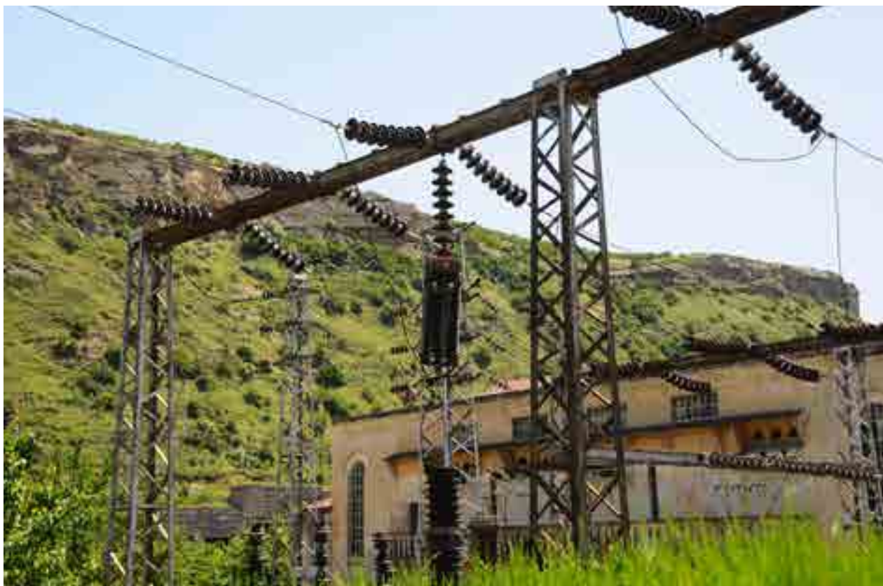
■ A sub-station of the Zahesi hydro power plant, the oldest in Georgia, reconstructed under the Black Sea Energy Transmission System project (Maia Edilashvili © EU/Neighbourhood Info Centre).
