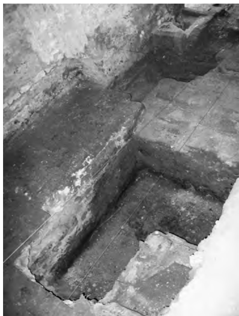
Fig. 11. The remains of an in situ frame or metal grid of the original air-heating system.
